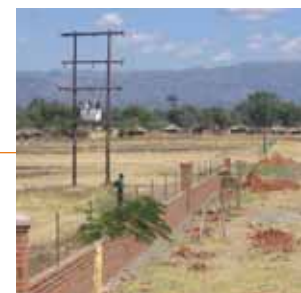
Transformer on Substation Poles
